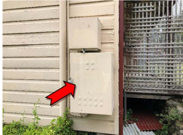
Photo 2. Exterior, southern elevation, electrical backing board – suspected asbestos-containing bituminous backing board.
