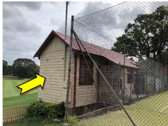
Photo 10. Exterior, throughout, walls – suspected lead-containing beige upper coloured paint system.
