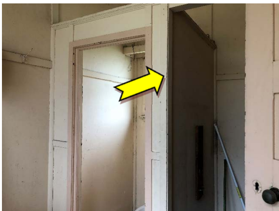
Photo 11. Exterior, throughout, windows and door frames - suspected lead-containing red upper coloured paint system.
