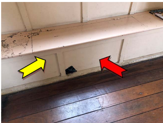
Photo 5. Interior, northern elevation, toilet, low level infill panel – asbestos-containing fibre cement sheeting and suspected lead-containing white upper paint system.
