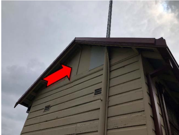
Photo 1. Exterior, northern and southern elevations, gable – suspected asbestos-containing fibre cement sheeting.
