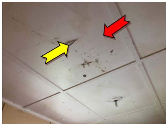
Photo 6. Interior, throughout, ceiling – suspected asbestos-containing fibre cement sheeting and suspected lead-containing white upper paint system.
