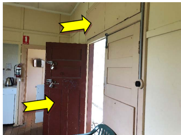
Photo 12. Interior, throughout, walls, windows and door frames – suspected lead-containing cream and pink upper coloured paint system.
