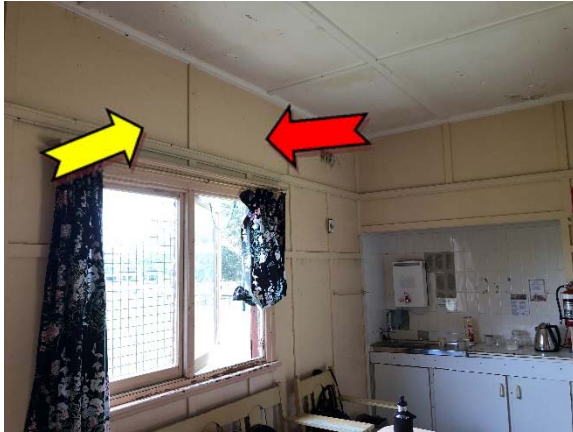
Photo 7. Interior, throughout, walls – assumed asbestos-containing fibre cement sheeting and suspected lead containing white upper paint system
