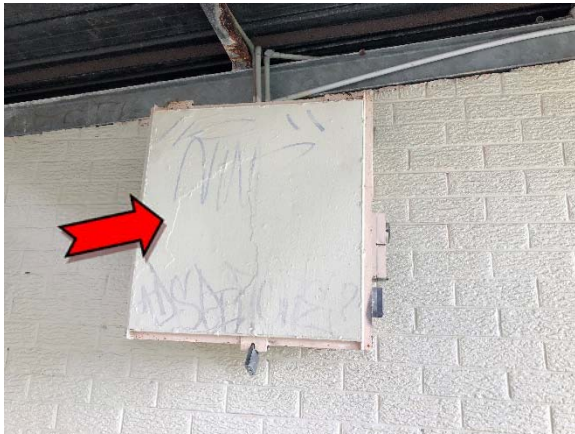
Photo 3. Exterior, northern elevation, electrical backing board – suspected asbestos-containing bituminous backing board.
